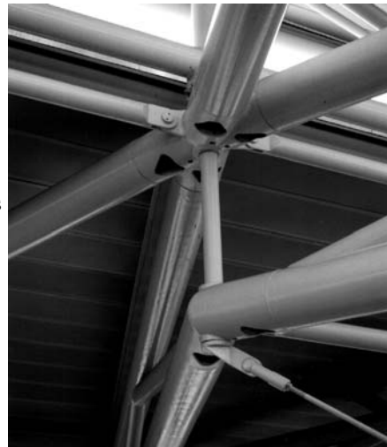
22 Structural steel castings connect diagrid members.
