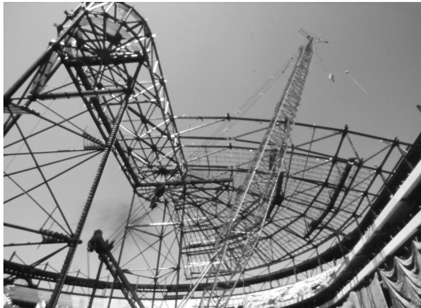
Figure 5: Marine Midland Arena Roof Construction. Shoring towers were used to hold the roof in its “weightless configuration.”
