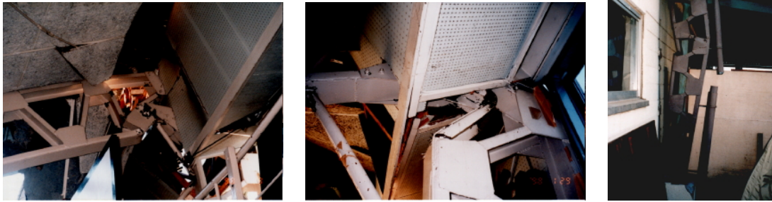
(a) End of the girder (b) Top of the column (c) Buckling of the column
