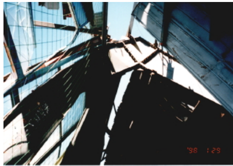
(a) Column torsional deformation
