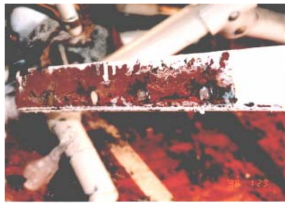
Photo 3: Shear cut of the center connection
