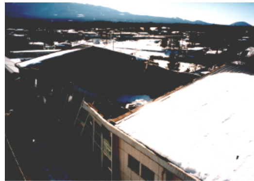
(b) After collapse
