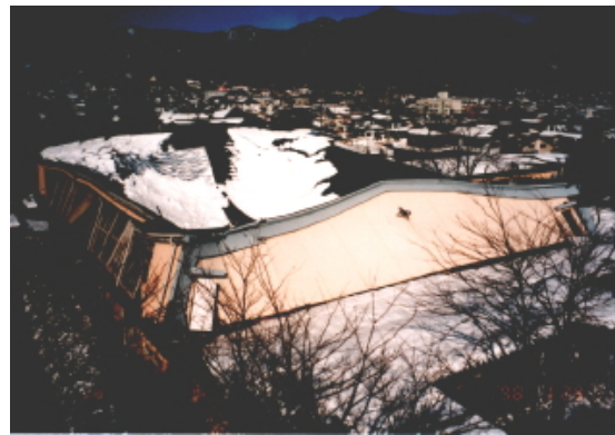
(b) After collapse
